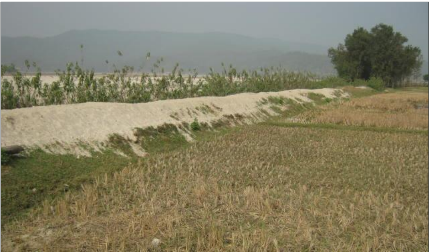
Picture 2: Sand embankment protecting paddy fields. Photo: Kenneth Bauer
